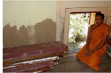
A few new buildings are under construction in the Wat Khun Samut's compound, resting on wooden and concrete pillars grouted into concrete slabs sunk into the mud beneath, which is under inches of water on a normal high tide. ST PHOTO: NIRMAL GHOSH
