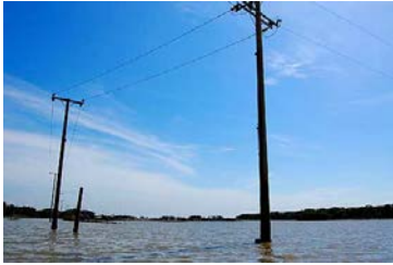
Telephone poles stand in neat rows out at sea, the brown waters of the Gulf of Thailand roiling about them. ST PHOTO: NIRMAL GHOSH
